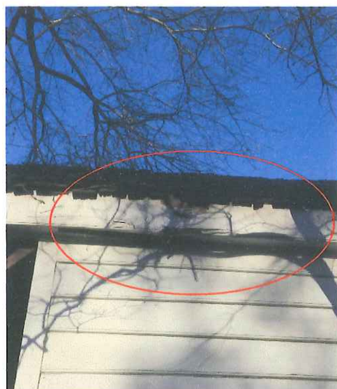
Advanced deterioration of the fascia and soffit.
